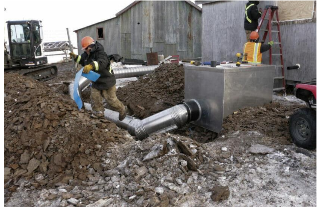
ANTHC workers install a water and sewer system to an Eek home on February 21, 2019. (Anna Rose MacArthur/KYUK)
