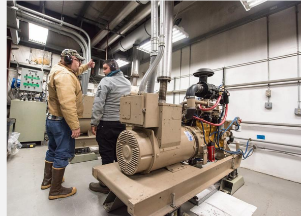
Daniel Rich, Mayor of Ouzinkie, leads a tour of the Village of Ouzinkie on Kodiak, Alaska. Diesel Power Plant. Photo by Dennis Schroeder, NLR
